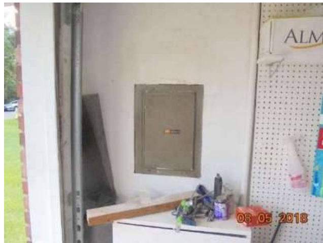
Photo 17-2 View of electrical panel.
